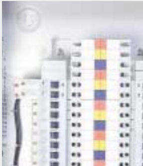
1 module RCBO's can be installed as outgoing devices
