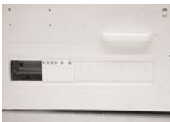
Insulated Tie Bar inside enclosure
