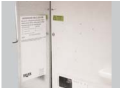
Underground Cable Location Sticker
