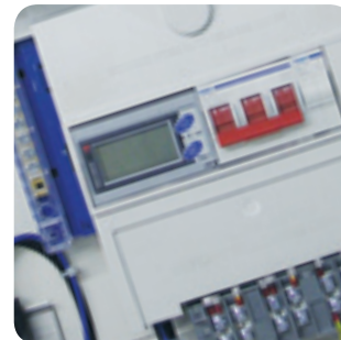
Metering fitted next to incomer within board
